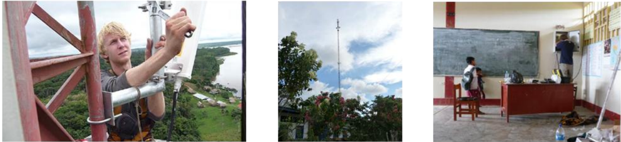
Figure 2: L-R (1) undergraduate researcher working on a tower; (2) network tower in Santa Clotilde; (3) undergraduate researcher installing a wireless router in the primary school in Campo Serio.
