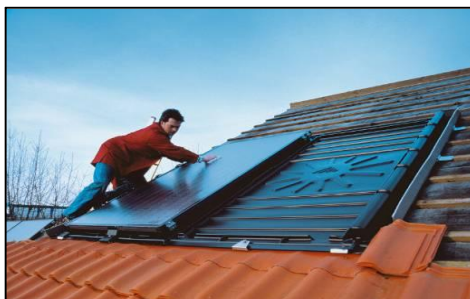
solar heating systems
